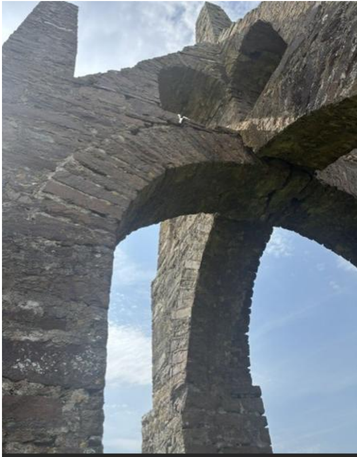
Picture taken at the Lacken Gazebo showing structural issue on the 26/05/26. Less than 300M from AT16 and 501M from the proposed Turbine AT15
