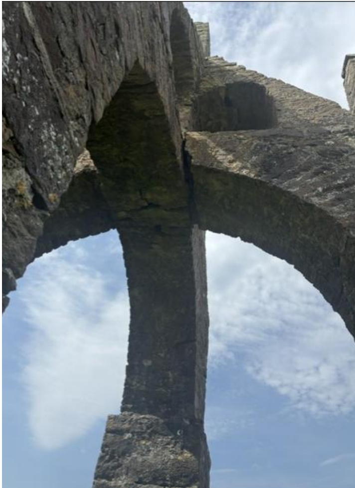
Picture taken at the Lacken Gazebo showing structural issues on the 26/05/26. Less than 300M from AT16 and 501M from the proposed Turbine AT15
