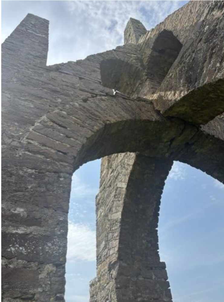
Structural issues on Gazebo picture taken 25/06/26
